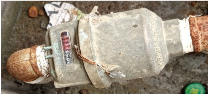
Water pipe meter
